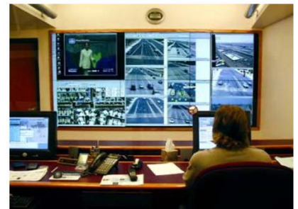
Figure 1: Large Display at Traffic Management Center
